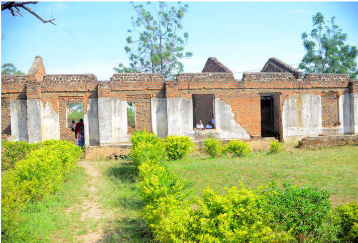
Before renovation: A dilapidated classroom block at Oreku Primary School in Arua, which was selected to benefit from proceeds of the NSSF Kampala Hills Run
